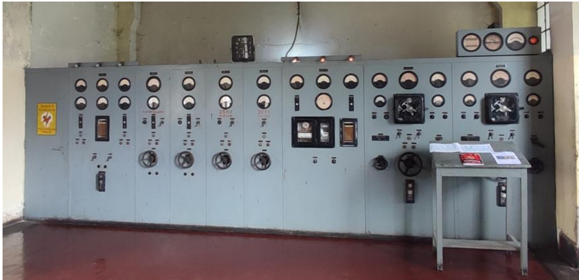
Figure 10. Switchboard at the Cijambe hydroelectric power station (Authors' Source).
